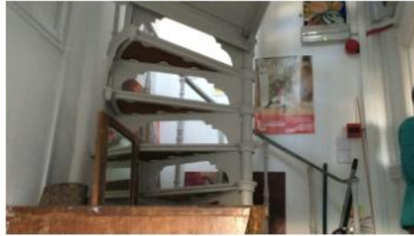
View of staircase leading to HMO studio apartments at 3rd floor level
